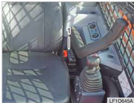
1) Cabin relay box
